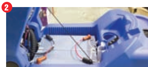
Compartment des batteries / Battery compartment
